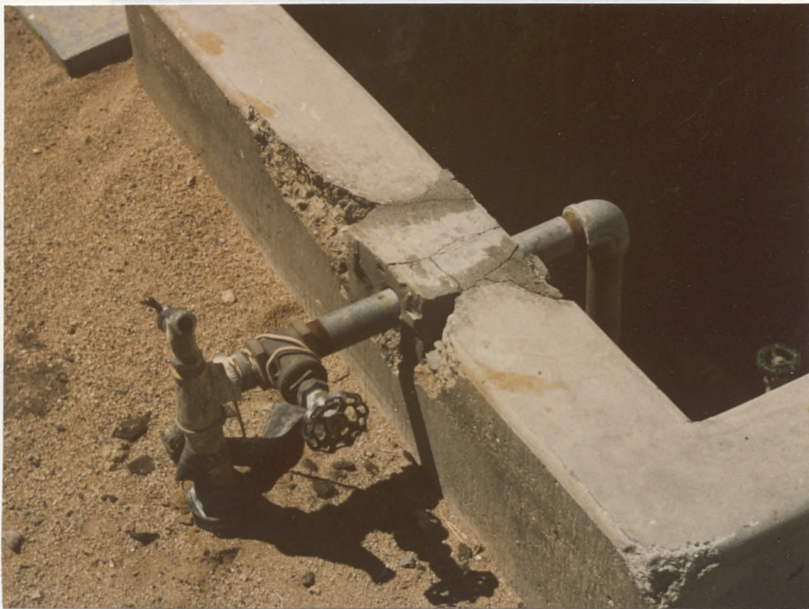
FIGURE 46. Water pipe and concrete retainer wall. The water pipe pulled from the concrete which was patched. Later, however, events have begun to remove the patch.
