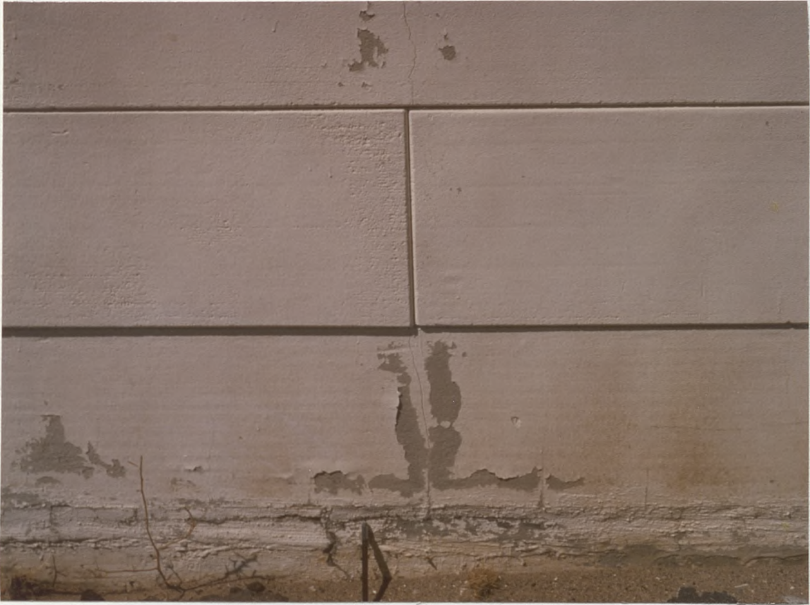
FIGURE 45. Closeup view of machine shop wall showing cracking and grouting along the foundation where the wall shifted about 2 centimeters off the foundation.
